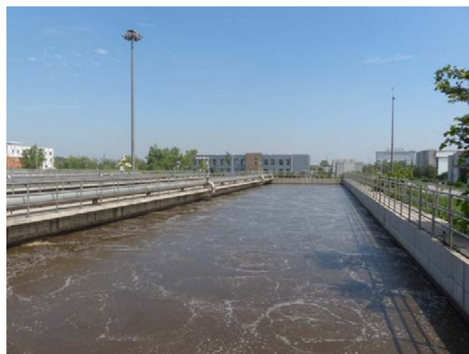
Weijia sewage plant, Beijing
